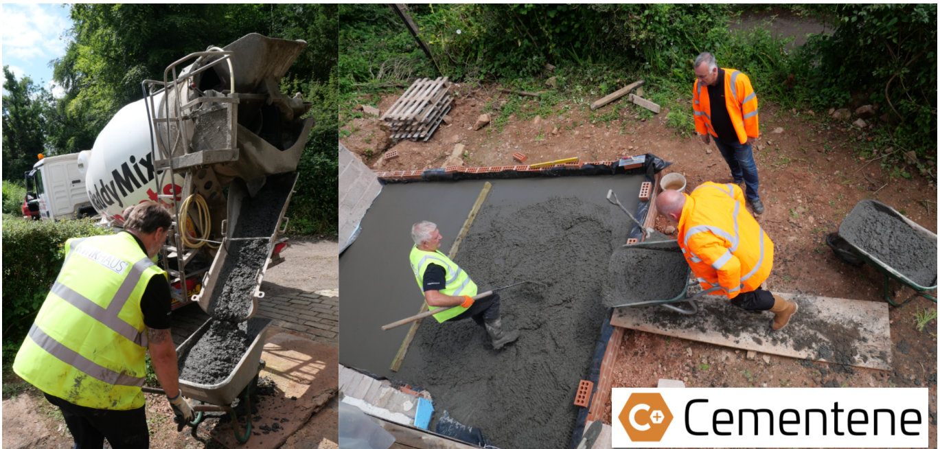
Fig. 7 Versarien's Cementene™ product being trialled on site in Symonds Yat, Gloucestershire, in collaboration with Kwikhaus UK Ltd.
