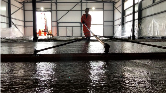
Fig. 8 Concretente™ slab laid in Amesbury, Wiltshire with 30% cement reduction and no steel reinforcement used. Credit: Nationwide Engineering Ltd.
